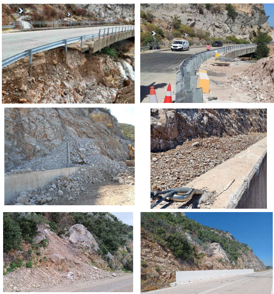
Figure 6. Characteristic views after the devastating heavy rainfall “Daniel” (left side) and restoration works (right side)
