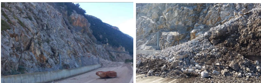
Figure 3. Falling of an individual boulder of 8m 3 (maximum boulder size of the rockfall) that bounced off the existing protection measures and ended up on the road deck within the provincial road, at about Ch. 5+525 km. Close-up view of debris flow (on the right)
