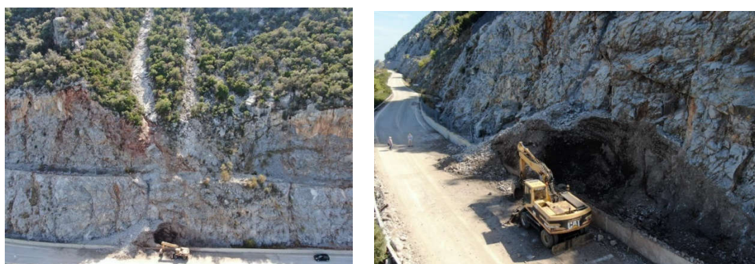
Figure 2. Debris cone and alluvial material at the base of the slope and within the road, from material accumulated through the two talweg - gullies.
